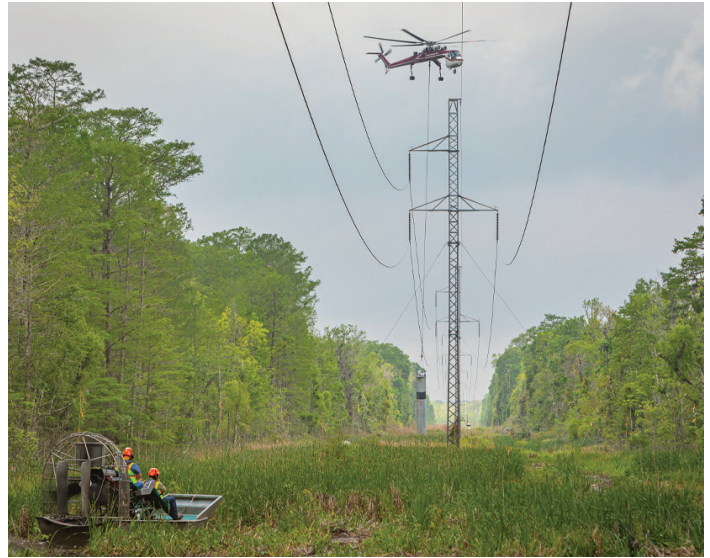
Figure 1: Building higher strand-count cables in some areas can be costly, due to logistics.
