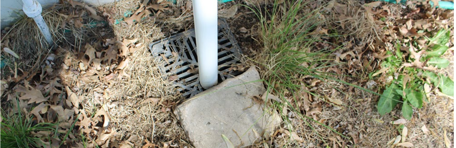
A sump pump is connected to an inlet that discharges water into the yard, facilitating proper drainage.
