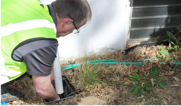
Keep Out the Rain personnel conduct an exterior property inspection to detect improper sewer connections.
